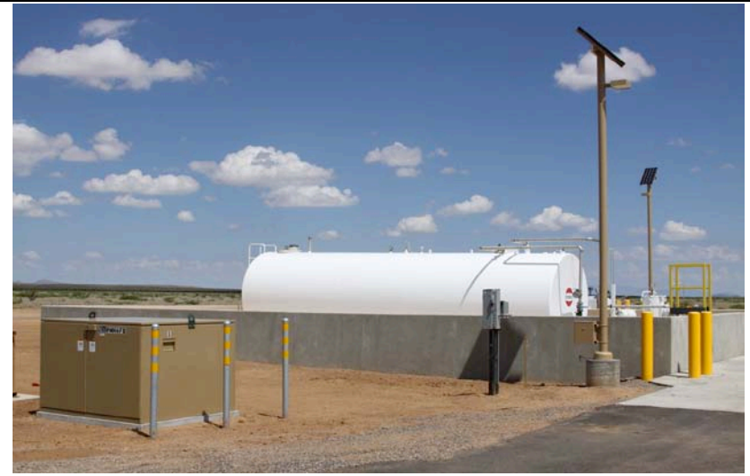
Fuel Storage Depot
