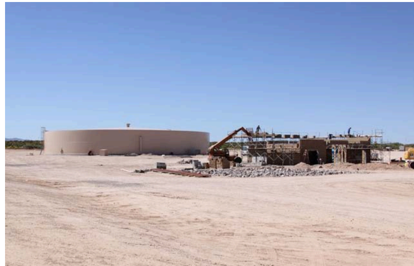
1.3M gal Water Storage & Booster Station
