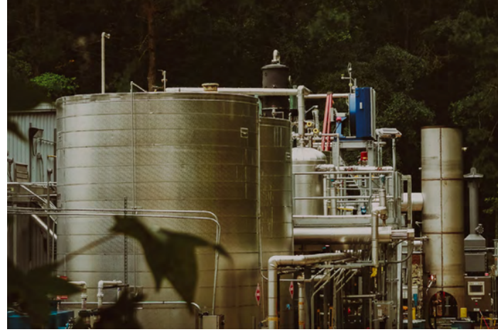
Braven Environmental facility in Zebulon, N.C.; courtesy of Schuyler Mitchell / The Intercept
