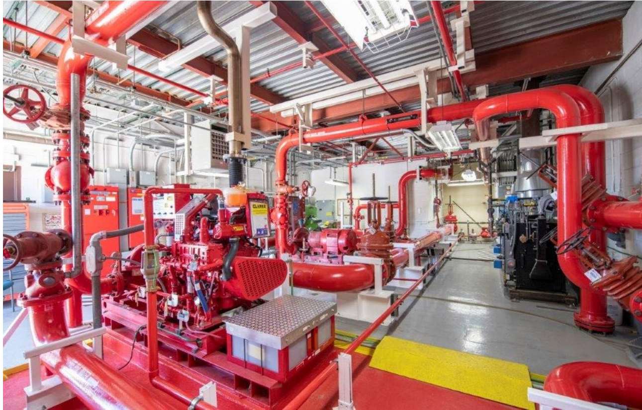
One of the firewater pump houses servicing the Plutonium Facility
