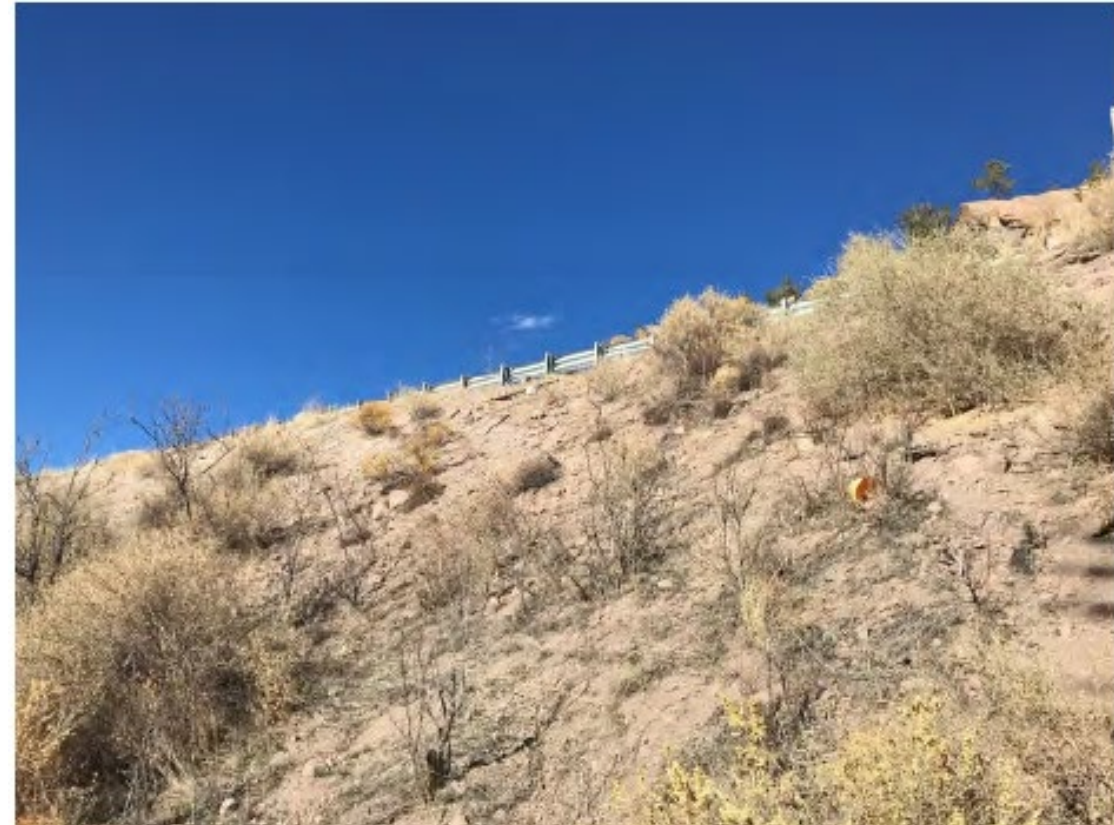
Cliff hazards along some Los Alamos roadways were not appropriately analyzed
