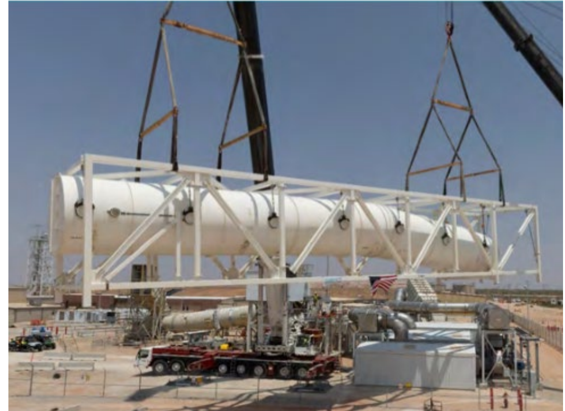
Installation of ducting supporting the Safety Significant Confinement Ventilation System at WIPP
