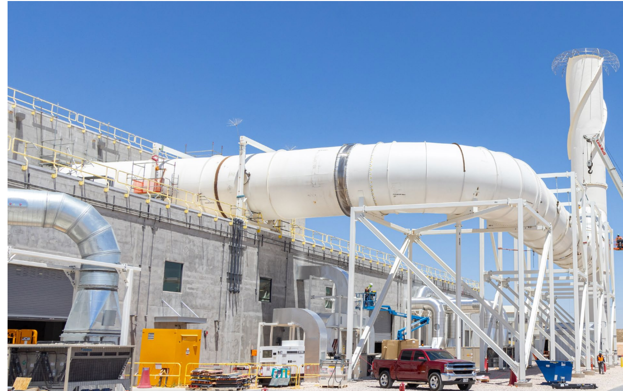
SSCVS filter building with exhaust duct and stack
