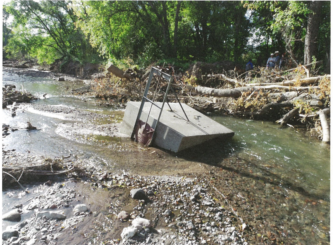
Above: Flooding from the Black Fire and impacts to the Grijalva Ditch Diversion in Grant County
