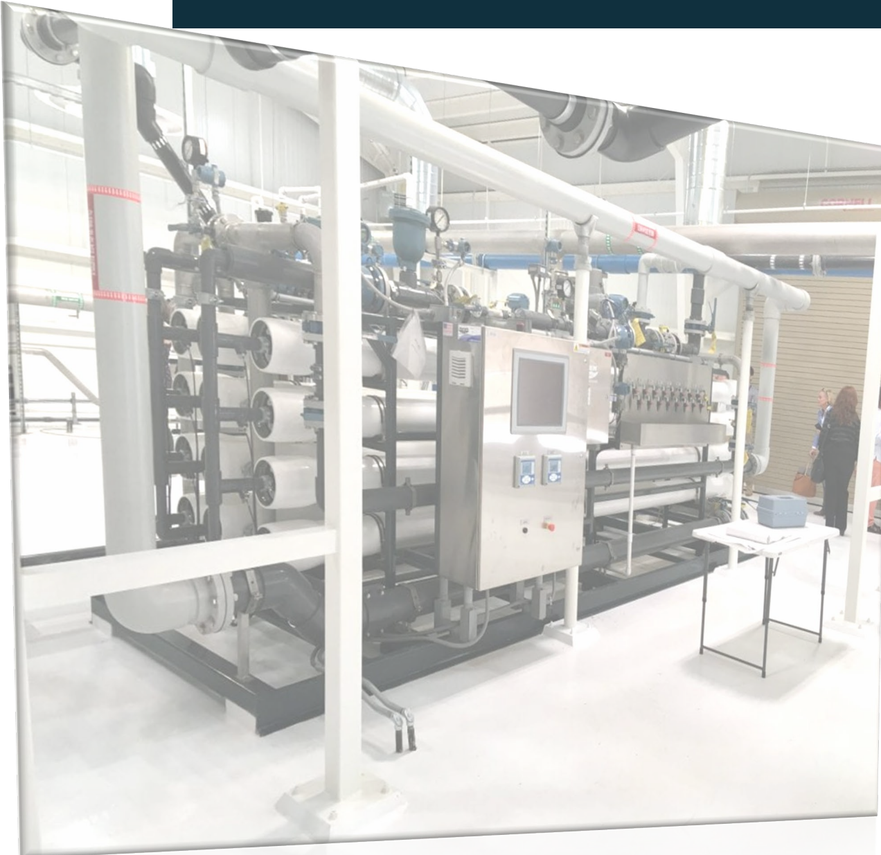
Desalination reverse osmosis skid in Alamogordo. Photo credit: Texas State University
