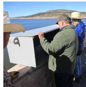
Control Box to Operate Pneumatic Valves Only one is operating.
