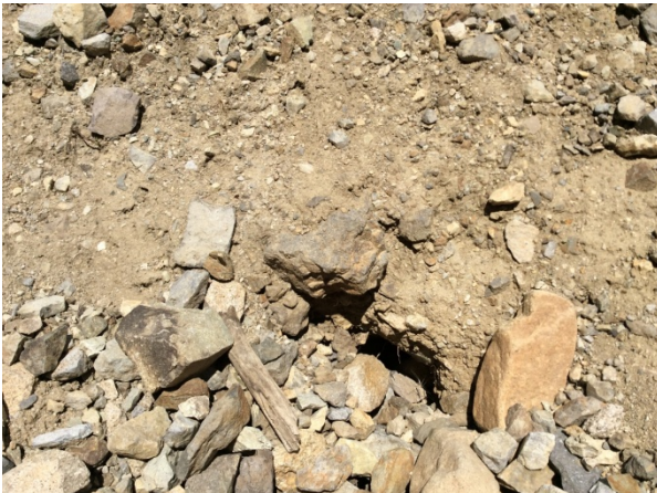
Suspected Seepage Hole
