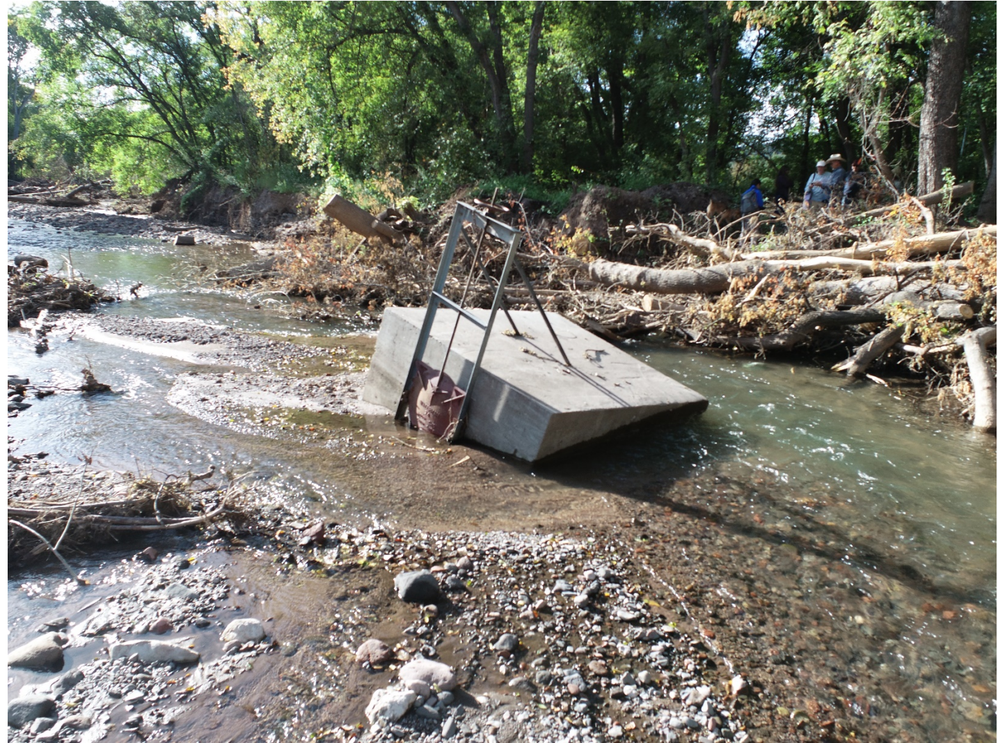
Above: Flooding from the Black Fire and impacts to the Grijalva Ditch Diversion in Grant County
