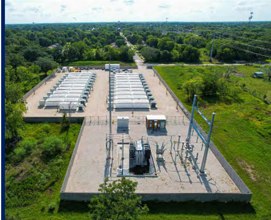
Gambit – Angleton, Texas In Operation
